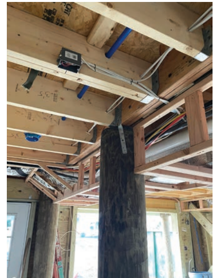
Some wind resistance details need to be completed on-site. For instance, the contractor has to install hurricane ties between the pilings and the home, between first-and second-story modules and between the modules and the roof.
