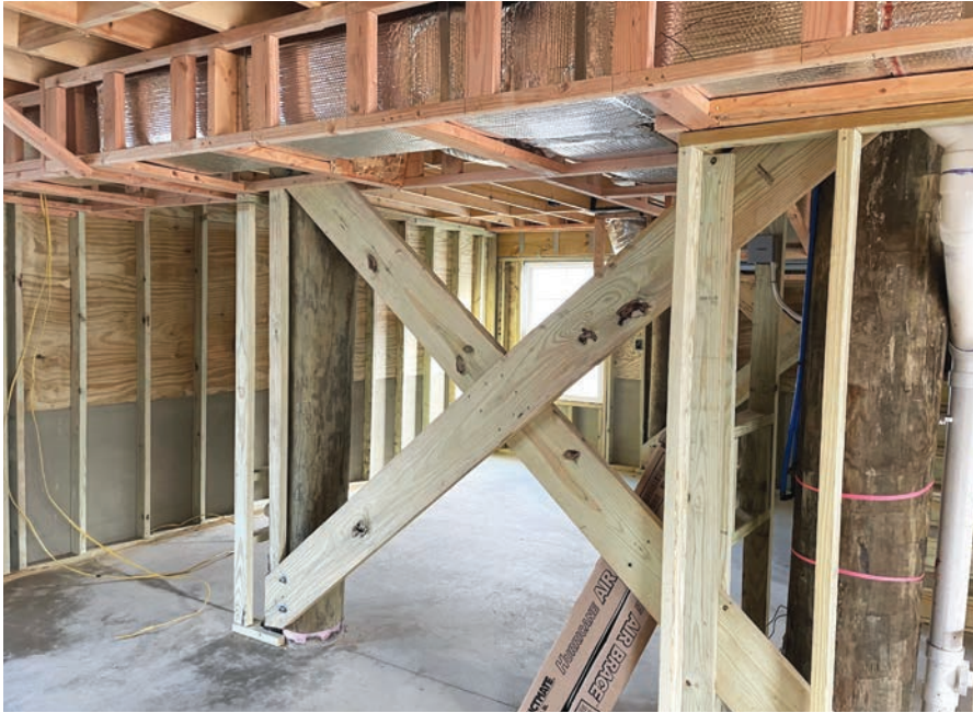
Although not required by code, the author uses diagonal braces to stiffen the foundation. This ensures the home doesn't move in even the strongest wind.
