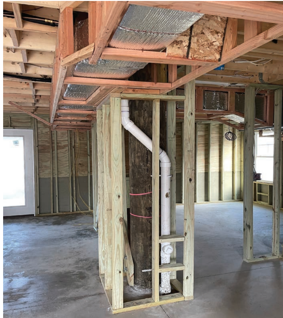
The area around a piling is a good spot for a plumbing drain.
