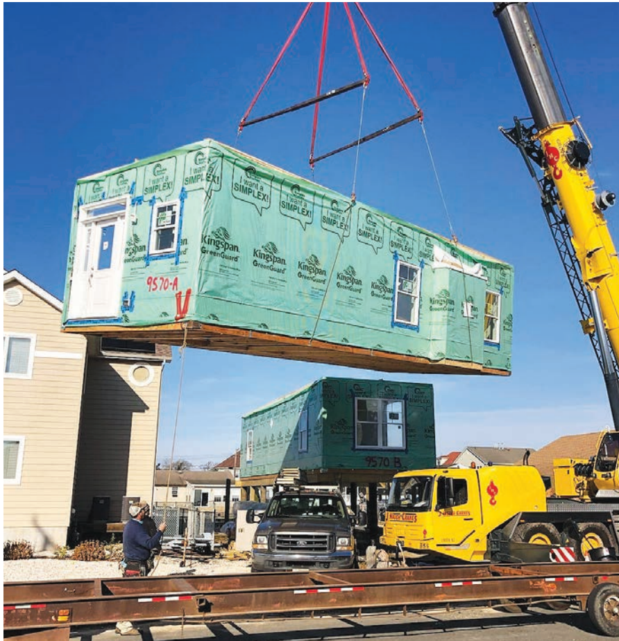
The factory engineers and assembles modules to the specifications set by local codes for wind resistance. For instance, roof rafters are secured to plates with hurricane clips.
